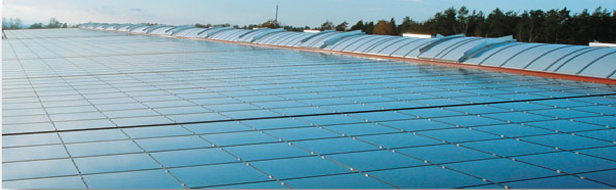
Figure 7.2: Thin Film Solar Array
